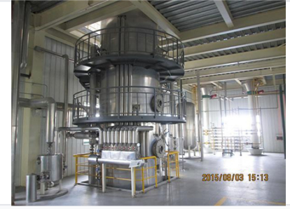
Deodorization tower designed for efficient odor removal and vacuum-based processing.
