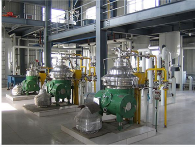
Degumming and Neutralization section featuring specialized reactors and separation units.
