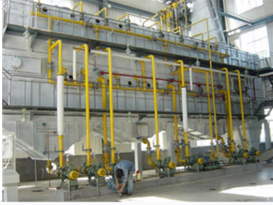
Complex piping and pumping arrangement for high-volume extraction.
