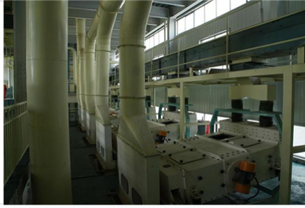
Cleaning and stone removal equipment integrated into the processing line.
