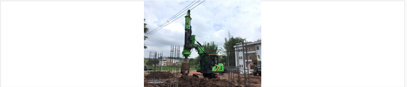
The rig is equipped with a versatile drilling attachment for precise pile foundation creation.
