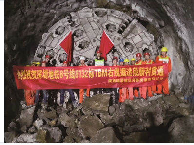
Successful breakthrough of a double shield TBM on a major metro line project.
