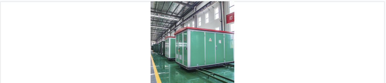
Compact design suitable for urban and industrial power distribution.
