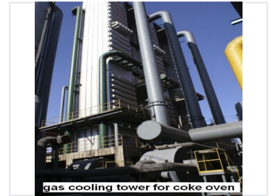
gas cooling tower for coke oven
