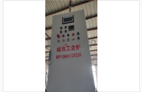
PLC-based control panel for intelligent, automated process management.
