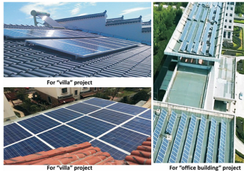
Successful solar power station projects from "QIXING"
