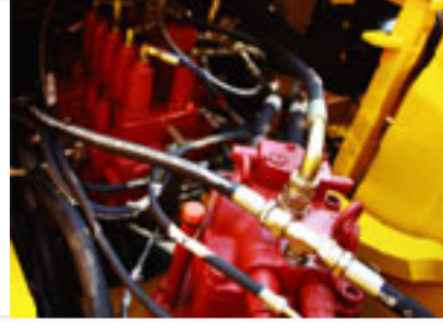
Intricate hydraulic network controlling excavator movements and functions.
