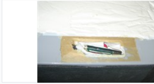
Built-in temperature transmitter for automatic seasonal adjustment.
