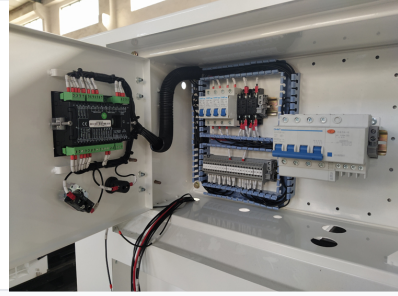
Internal electrical cabinet featuring MCBs and RCCB for comprehensive circuit protection.
