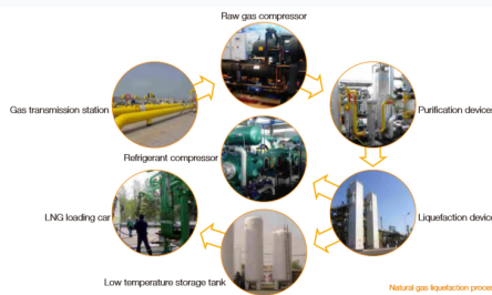
A detailed layout of the natural gas liquefaction process, highlighting the flow from transmission to final loading.
