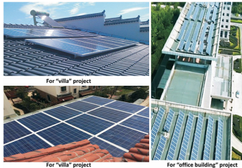
Successful solar power station projects from "QIXING"
