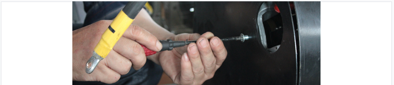
Detail of high-current electrical cabling and terminal connections during the assembly process.
